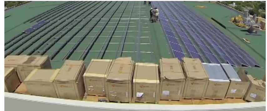
South America | 400 kWp
