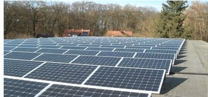
Ulzen, Germany | 50 kWp
